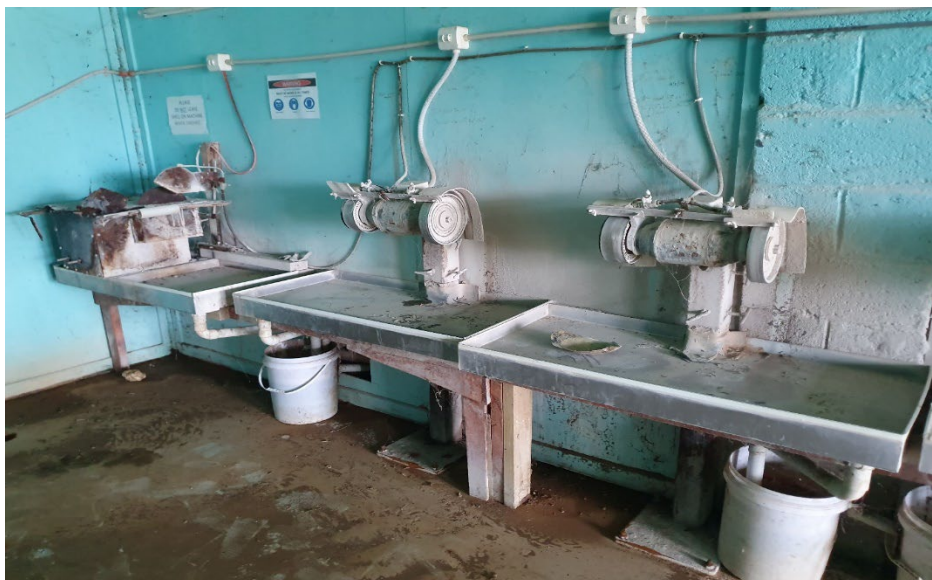
Broken power tools within the Vava'u Pearl Centre following floods in December 2022 which caused major damage to the training facility.
