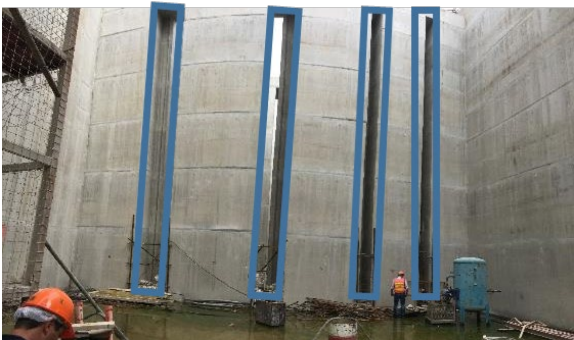
Figure A2.1. Slots where antennas were installed in the Xayaburi fish pass (source: unknown).
