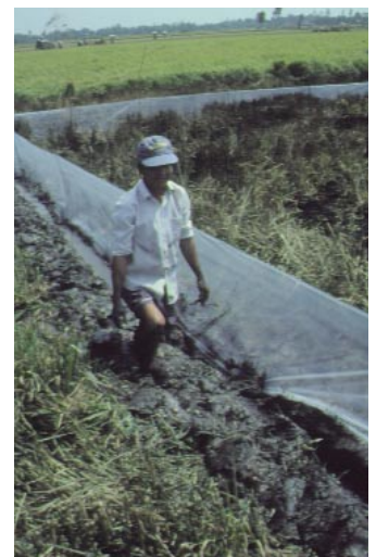
A CTBS under construction. The plastic must be dug 10 cm into the soil to stop rats crawling under the fence.
