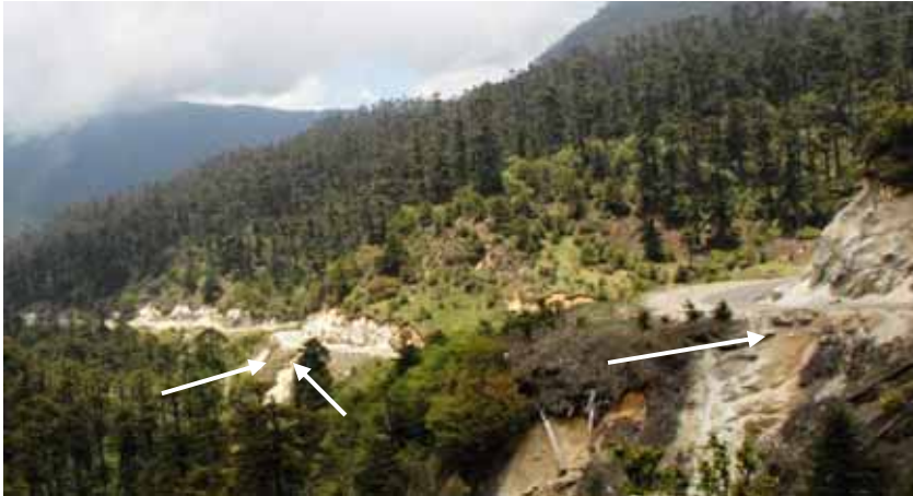
Figure 5 Soil erosion resulting initiated by road construction in sub-alpine forest (see arrows)
