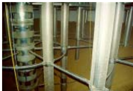
Filling the silo with rice during testing of the vertical air distribution system in the Mishan Grain Depot
